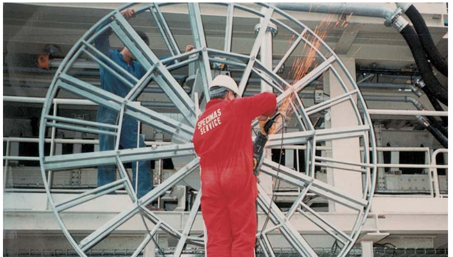
The commissioning of a giant hose reel for Madrid metropolitan tunnel drilling.
