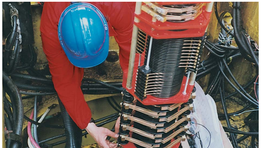
Replacement of a damaged slipping unit on an offshore application in Qatar, at +48 deg. C
